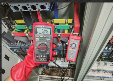
Bus bar current test
