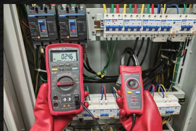
Power distribution box Current measurement
